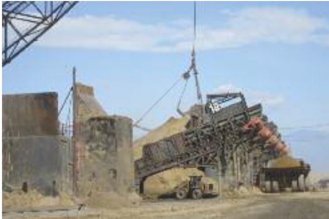
Draglines are used to load MMD feeders with overburden at Drummond, which in turn load the trucks. This shows the feeders at the Descanso pit. The apron feeders allow the trucks to be loaded very accurately in terms payload; also the loading technique of the feeder ensures the load is well balanced in the centre of the truck bed, which helps reduce tyre wear
